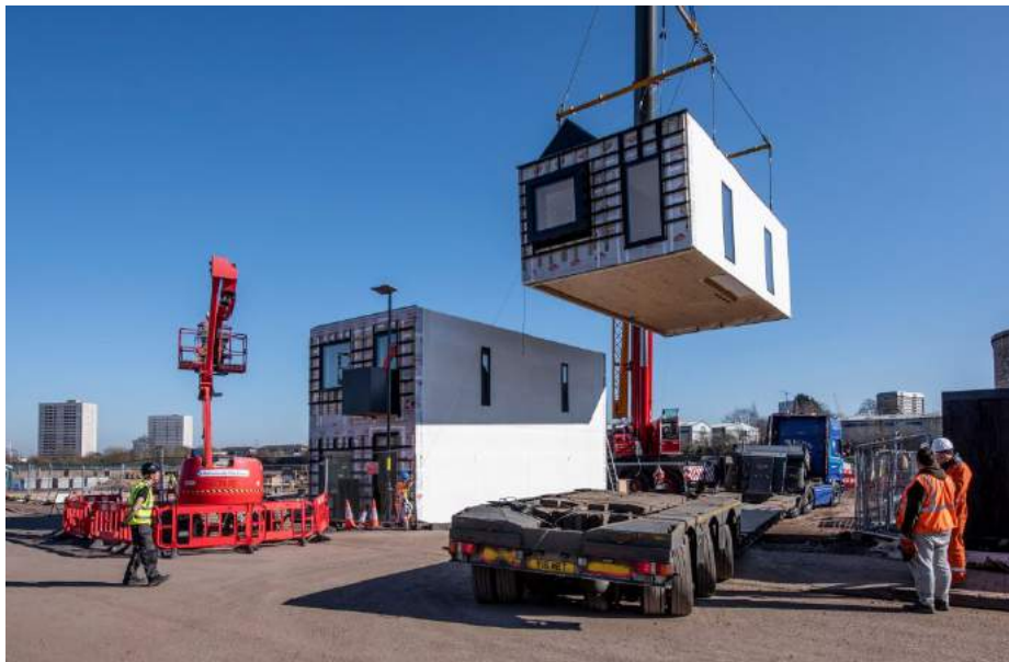
Figure 8: Image of modular homes being craned into place. (Source: Moore, K. (2019) [Online] [Accessed 10/10/19] Available from: https://www.birminghamupdates.com/first-of-40-modular-homes-installed-at-icknield-port-loop/ )
